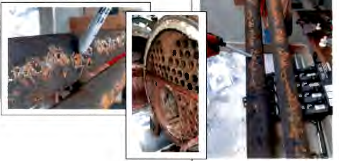
Fig.3: Removed fire tube showing extensive corrosion.
