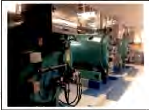
Fig.1: Boilers with their original burner configuration.
