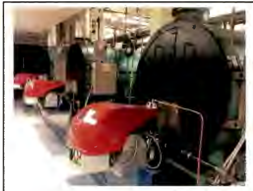
Fig.2: CB boilers fitted with door conversions and Riello burners.
