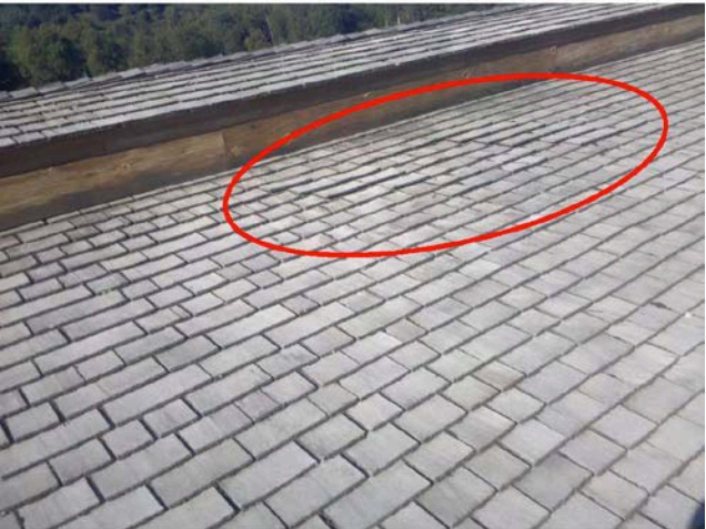
Shingles curling and cupping.
