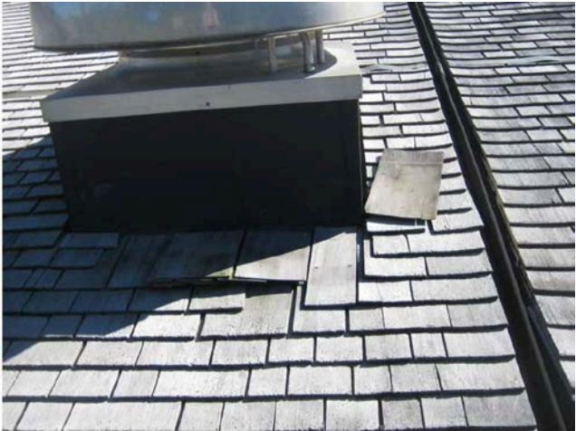
Shingles broken and sliding out of position.
