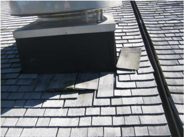
Shingles broken and sliding out of position.
