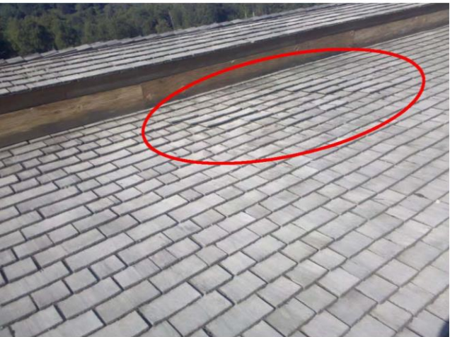
Shingles curling and cupping.
