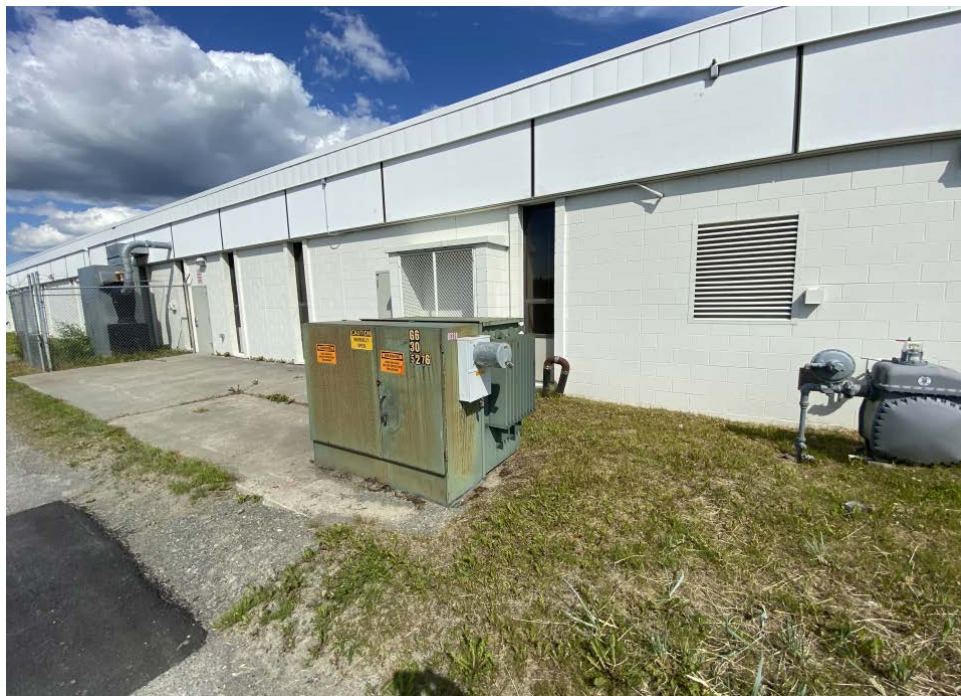
Main power service on west side of school
