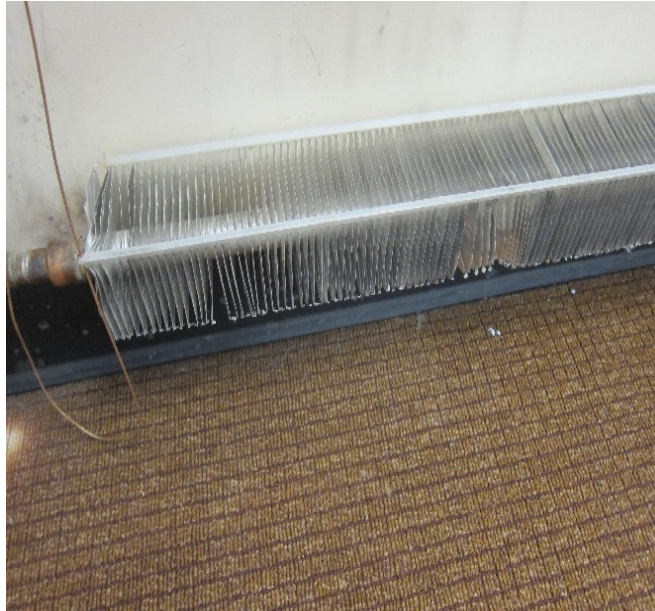
Classroom finned tube exposed with bent fins
