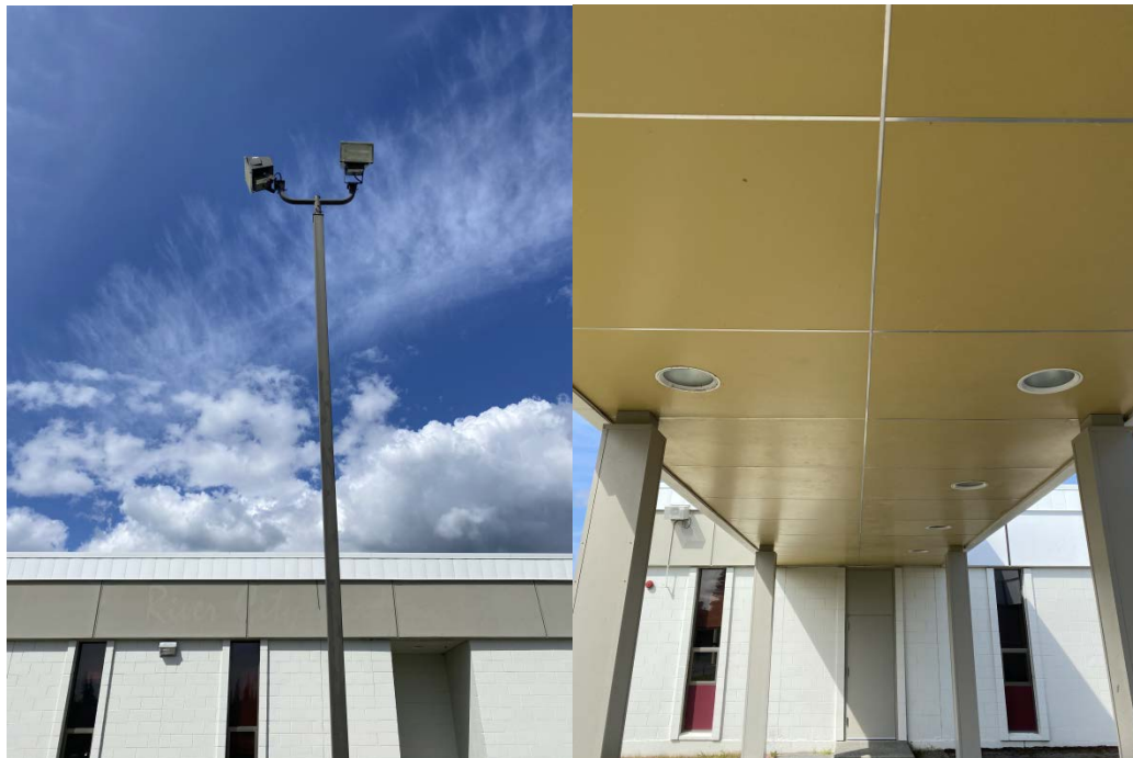
Pole lighting near front and front canopy lighting
