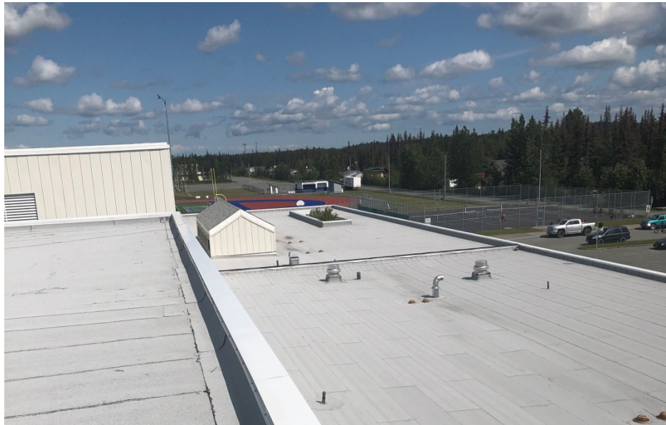
The roof of the school was replaced five years before the date of this report.
