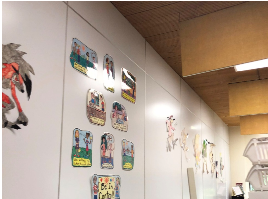
Pairs of classrooms are separated by operable partitions that can be manually opened.
