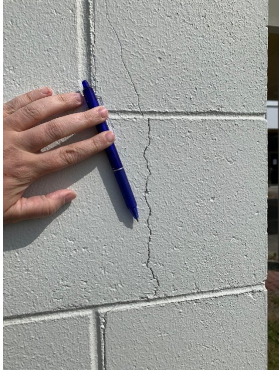
Enlarged view of cracking in CMU walls
