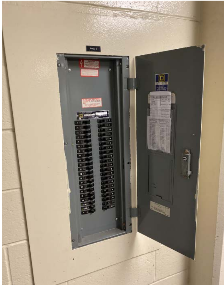
Example panel in hallway (no spares or spaces)
