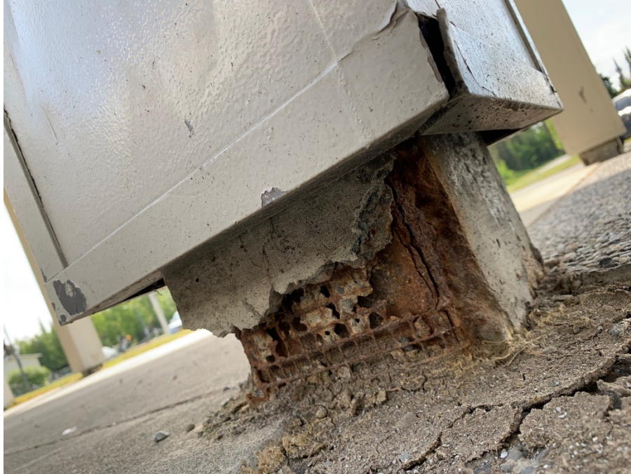
Typical damaged column base at school entrance
