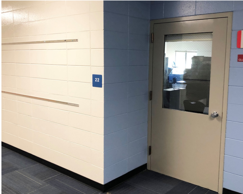
The doors along the main hallway do not have ADA compliant lever style handles.
