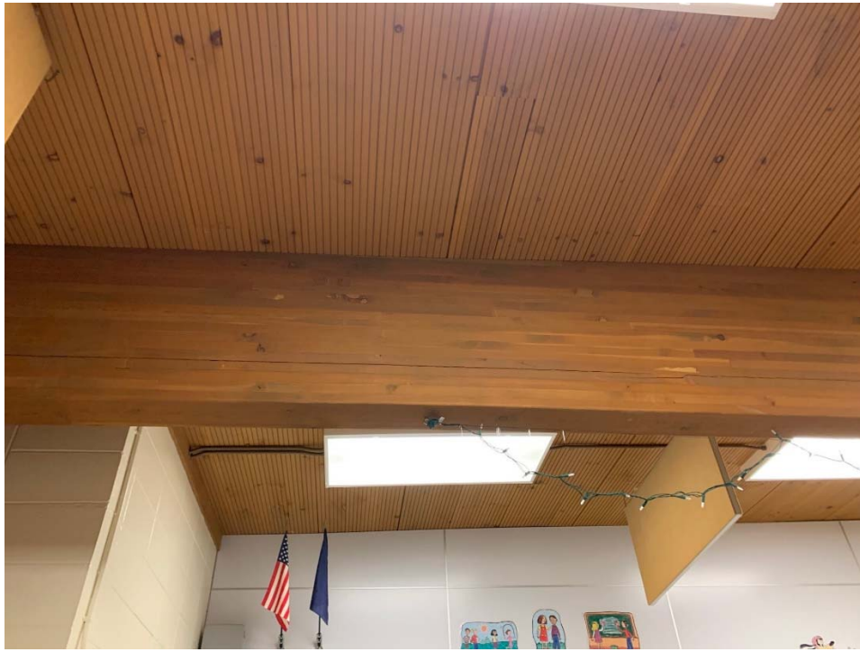
Poor fit-up in tongue and groove deck
