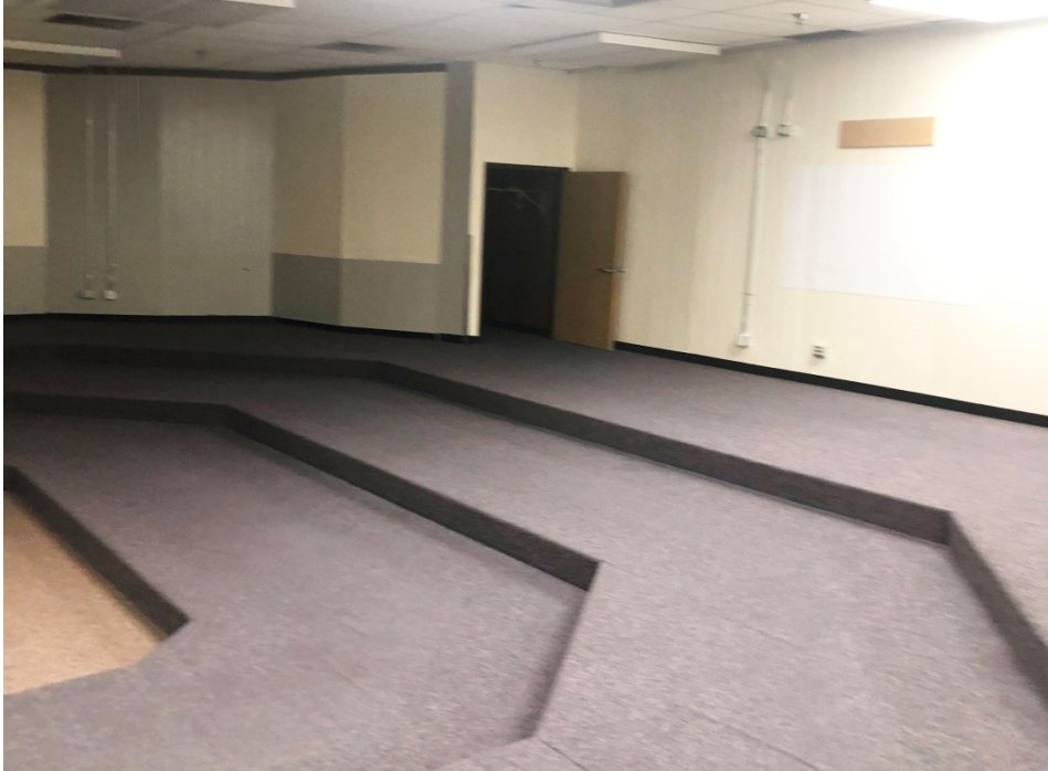
The tiered seating in the main music room/band practice space is not accessible.
