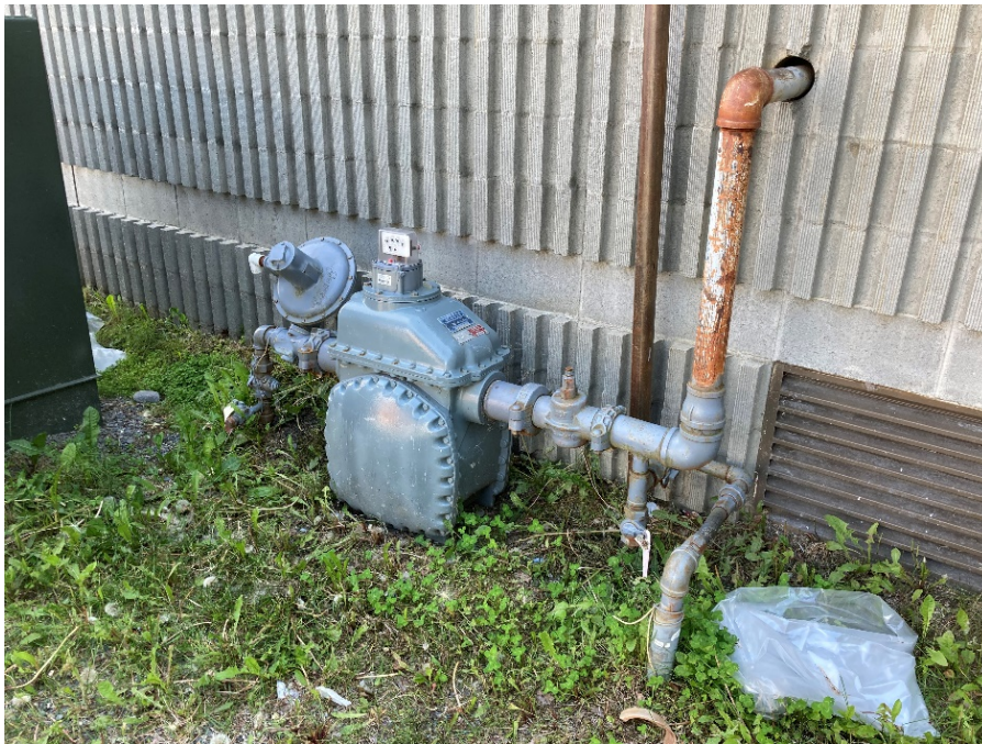
Gas meter at rear exterior of school
