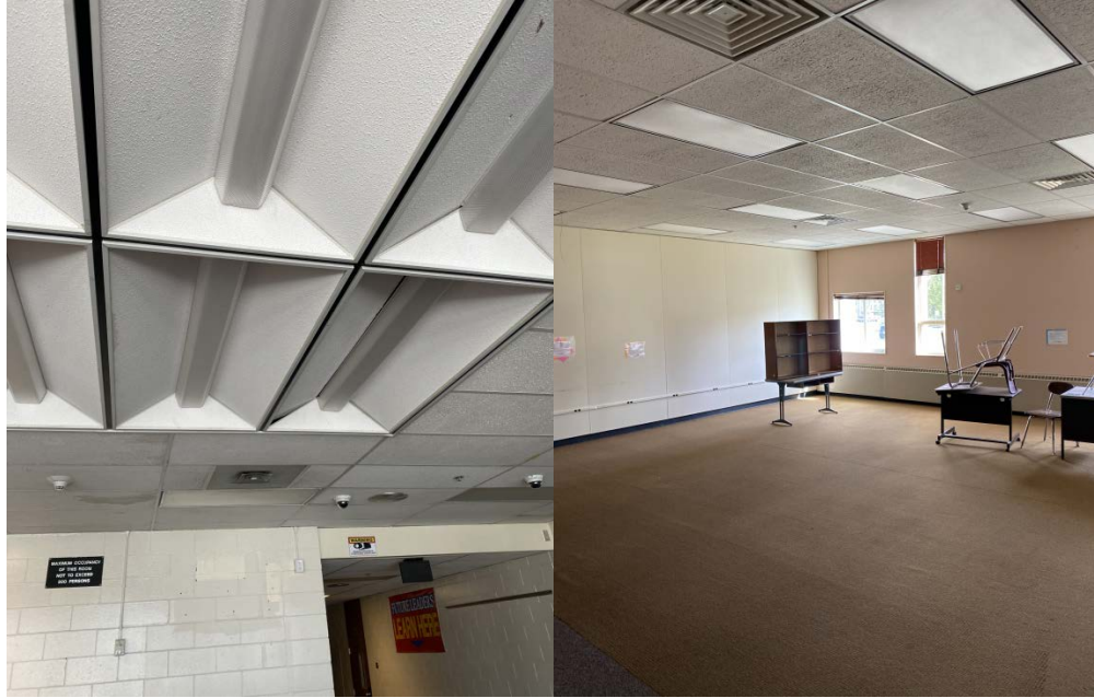
Lighting near front entry and typical classroom lighting
