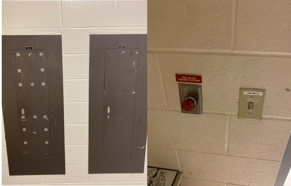
Shop panels and emergency shut down button in shop office
