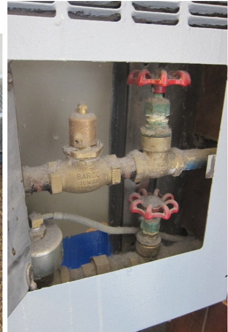
Terminal unit valves and piping in aging condition with pneumatic control valves
