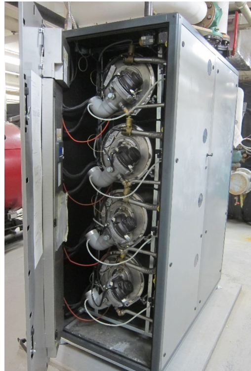
New boiler installed in 2017
