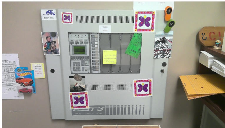
Redoubt main fire alarm panel in reception area
