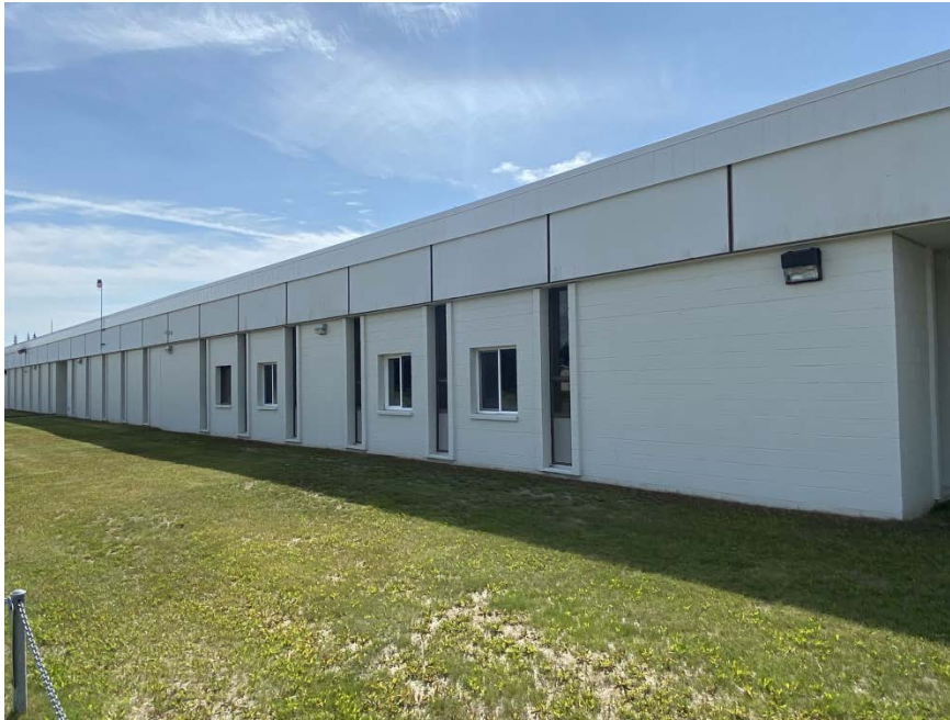
Wall pack lighting on east side of school
