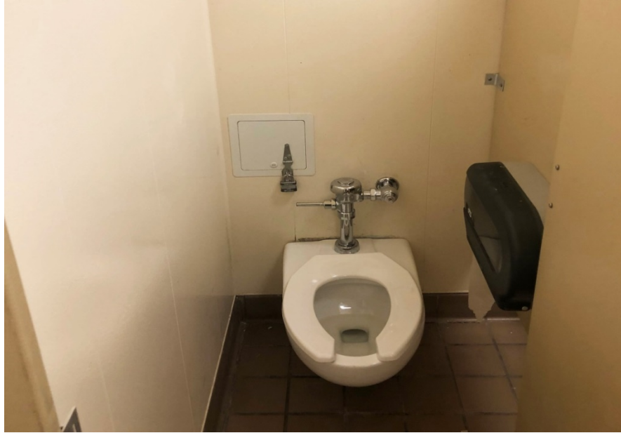
Neither the boy's or girl's restrooms in the south end of the building complies with the ADA guidelines for layout or fixtures.
