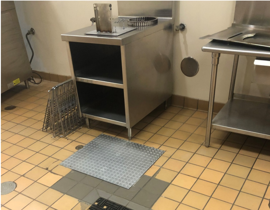
The tile base in the kitchen is chipped or cracked in a few locations.
