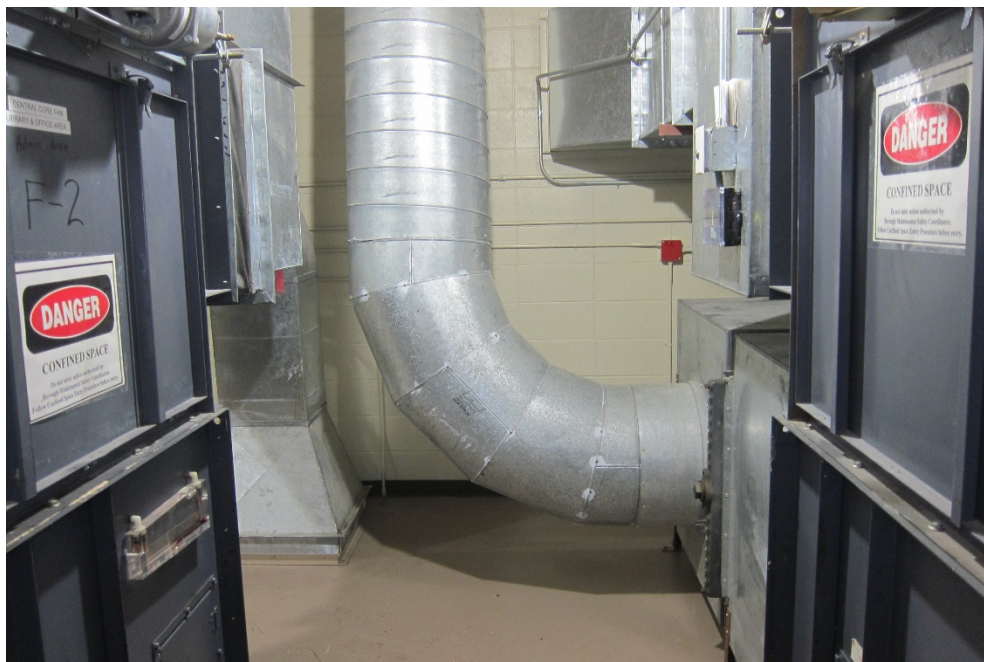
Multiple fan units are original construction
