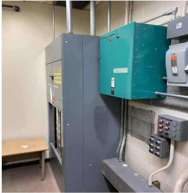
Main Distribution Panel and ATS
