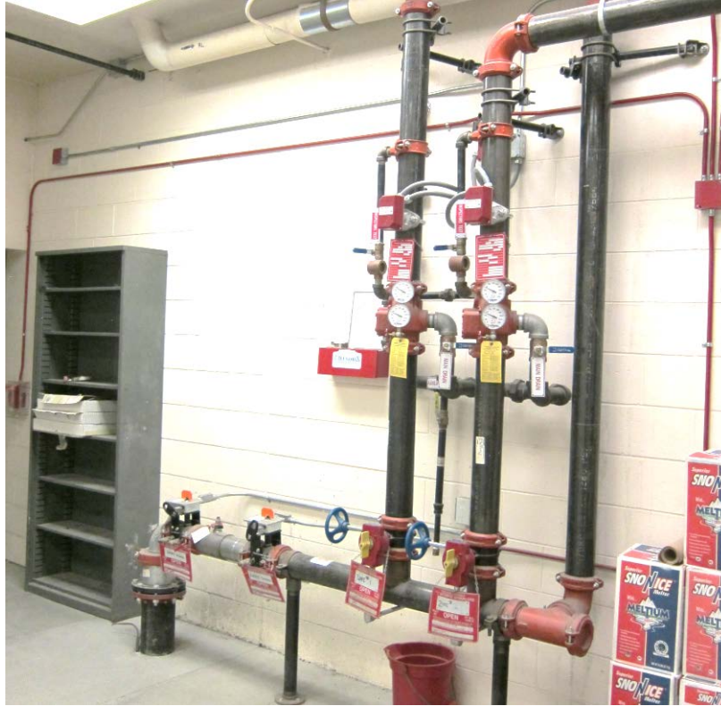
Fire riser with two zones in fire sprinkler room
