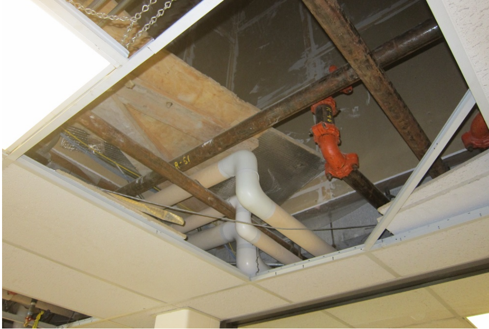
Piping conditions above ceiling with external corrosion and missing insulation
