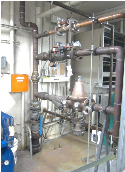
Water entry in boiler room
