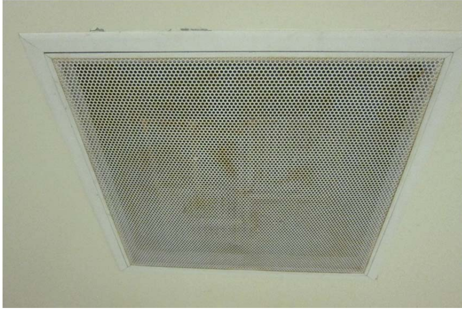
Ventilation grilles and diffusers require cleaning
