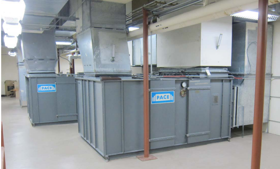
Fan units are all original installed equipment
