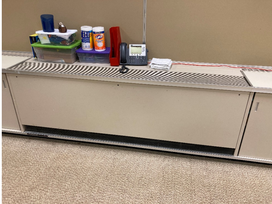
Fan coil units built into classroom cabinetry
