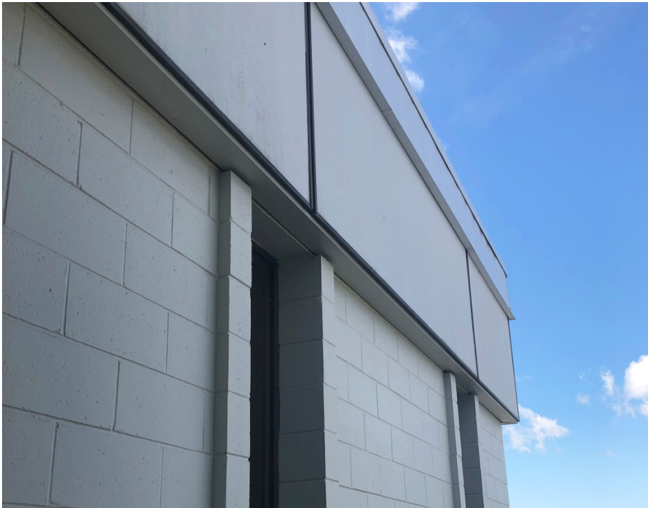
The exterior CMU is in good condition and shows no signs of damage.
