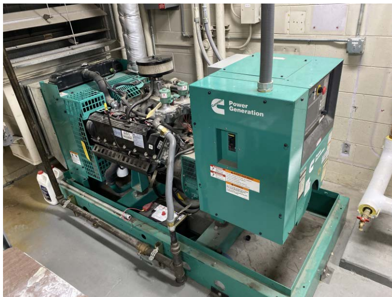
Backup power generator
