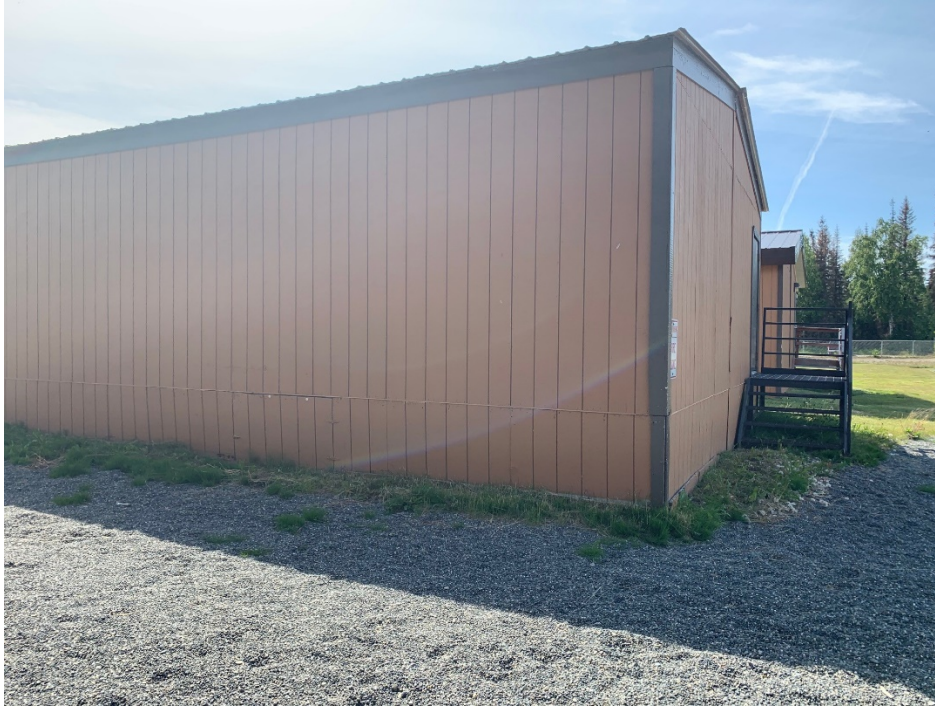
Portables in poor condition
