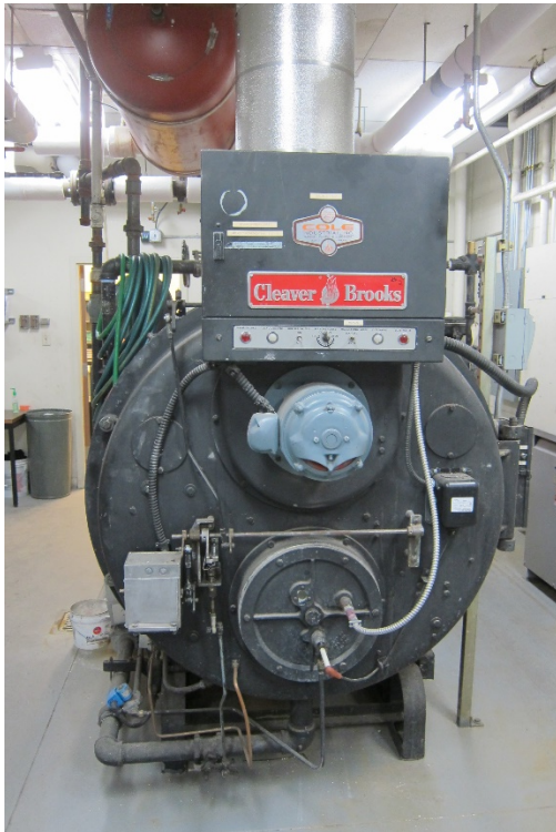
Older fire tube boiler at end of life
