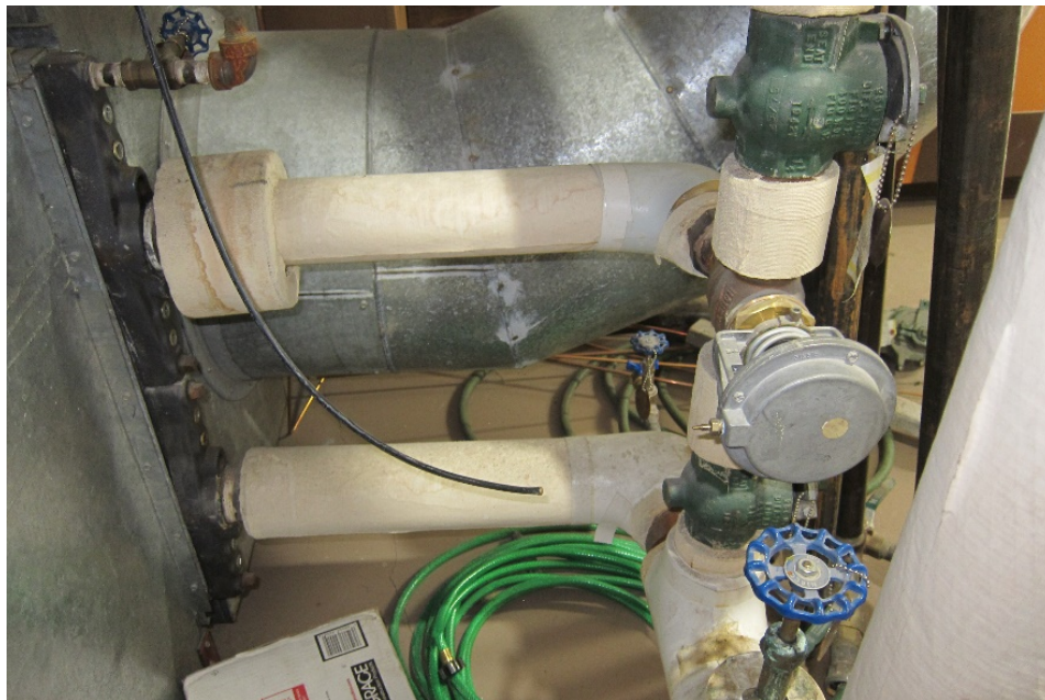
Air unit heating coil piping with pneumatic line disconnected
