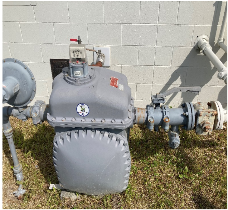
Gas meter on west side of school
