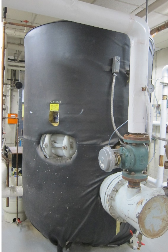
Water heater in boiler room
