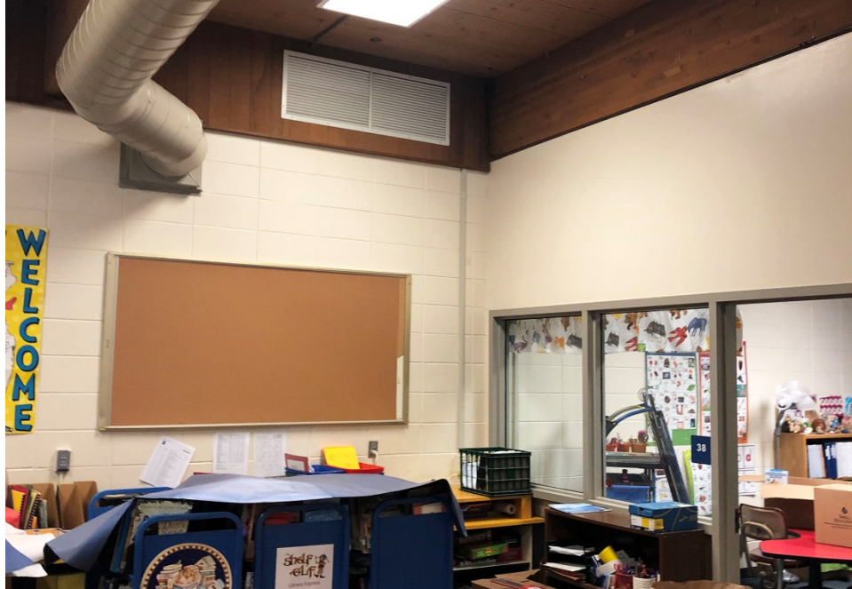
The library is a large double height space open to structure above.
