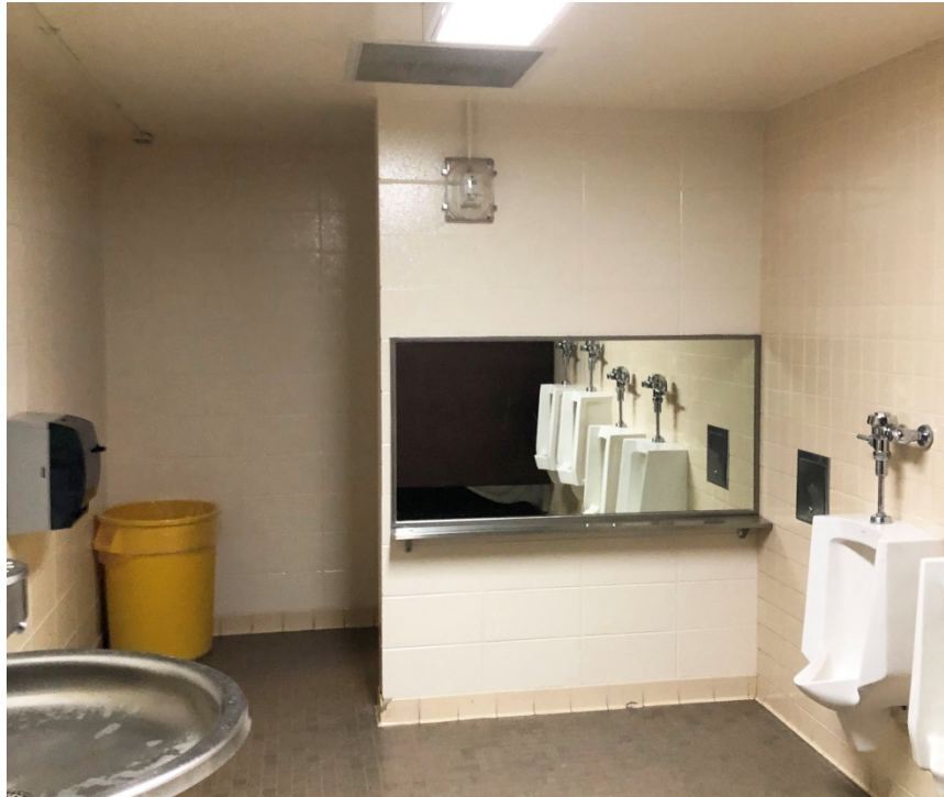
The restrooms are showing signs of wear and do not have ADA compliant toilet stalls.
