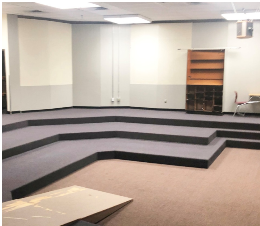
The tiered performance area in the music room does not have an accessible means of access.
