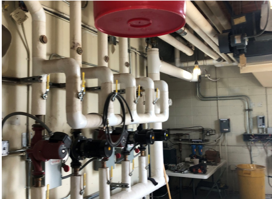
A view of the main boiler room.
