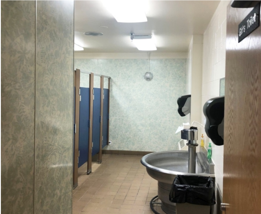
Restrooms in the south half of the school typically have some ADA accessibility issues.
