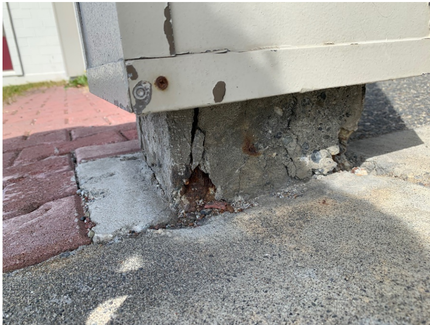
Typical damaged column base at school entrance
