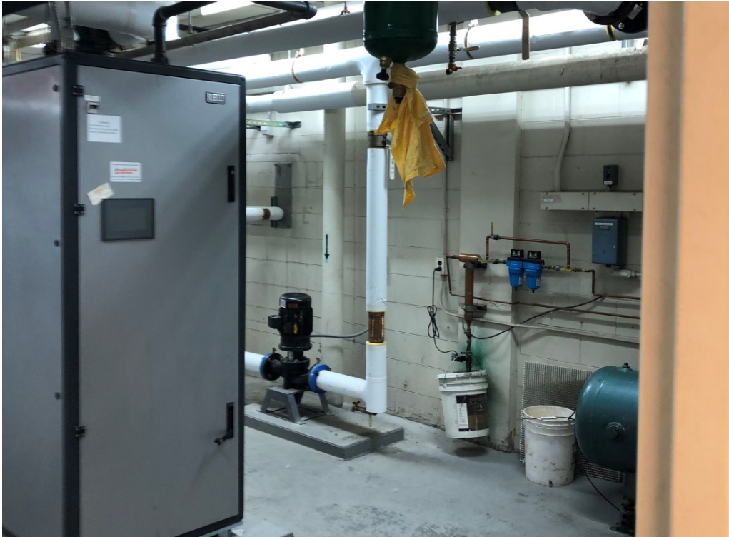
The main boiler room is clean and well maintained.
