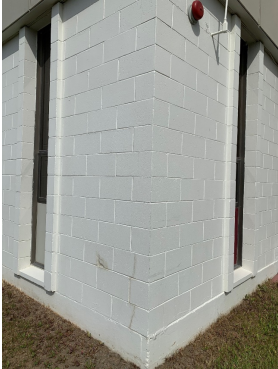
Cracking in exterior CMU walls
