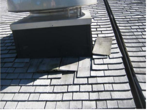
Shingles broken and sliding out of position.
