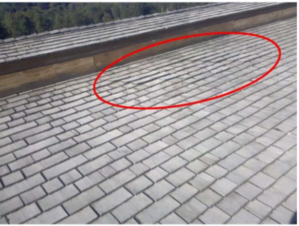
Shingles curling and cupping.
